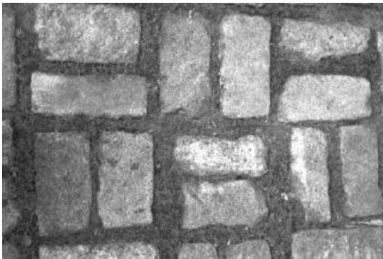
Uni-green Pavers for Fire-lane
